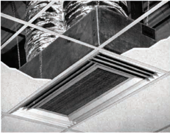
Light Commercial T-Bar Ceiling
