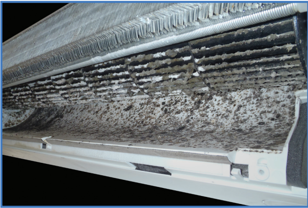
Mini-Split blower with MOLD
