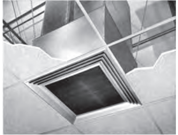
Commercial T-Bar Ceiling
