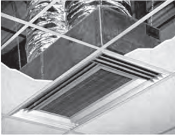
Light Commercial T-Bar Ceiling
