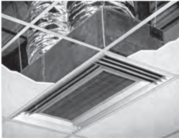
Light Commercial T-Bar Ceiling
