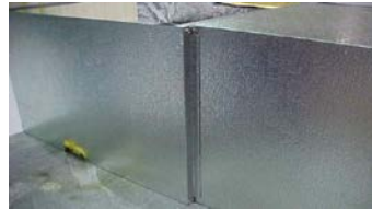
Back of HD coil (left) connected to a blower (right).
